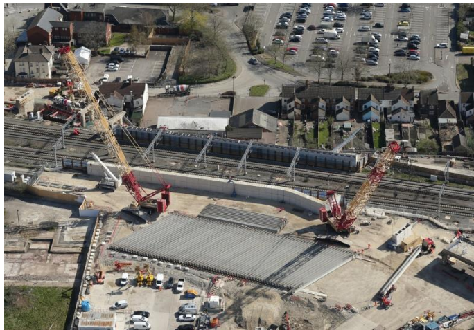
EWR construction.jpg EWR's Route E strikes through the heart of residential Bedford with six tracks and blunders on with four tracks into Cambridge
